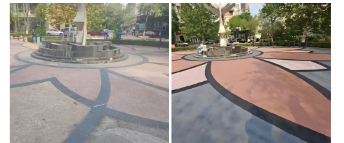
▲ 大連東城天下老舊廣場地面煥新升級 Outdoor Ground Renovation and Upgrade at Dalian Dongcheng Tianxia
